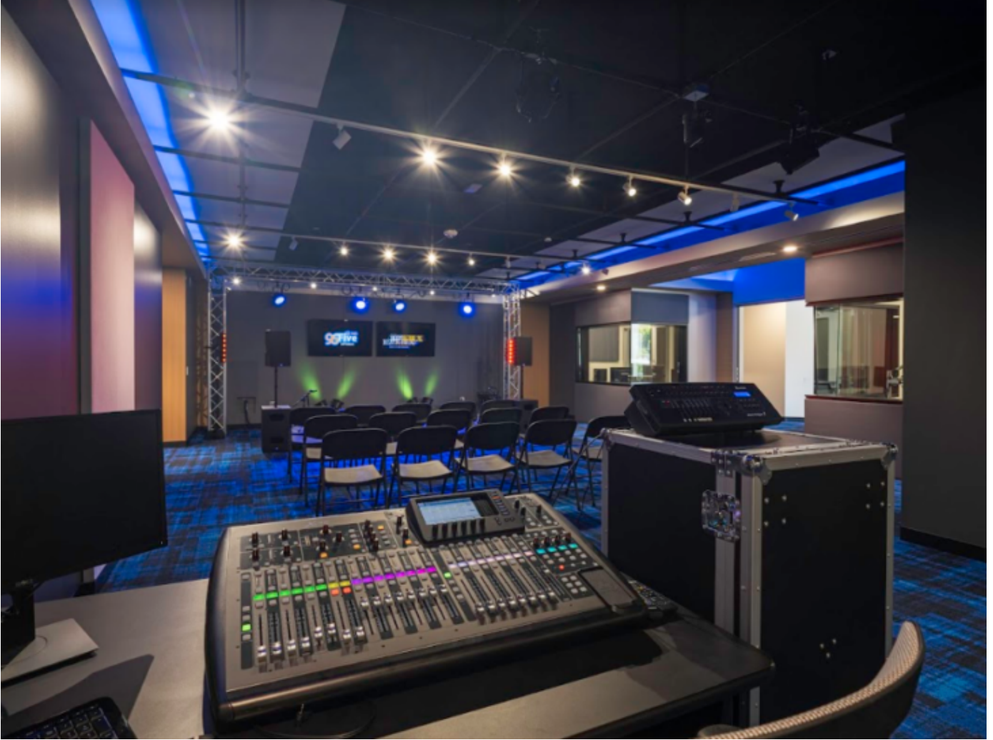
The performance space and adjacent audio and video control rooms.
